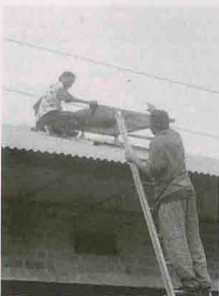
Cleaning of a photovoltaic panel during a maintenance tour at the health centre for Sundi Lutete, region of Bas-Zaire, July 1991
