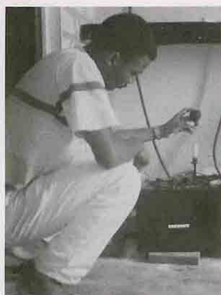
Measurement of the state of charge of batteries at the community battery photovoltaic charger system of Nselo, region of Bas-Zaire, August 1991.
